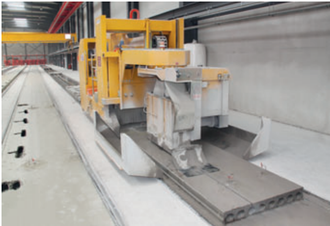
Longitudinal cutting on a cured hollow core slab carried out by Nordimpianti's multi-angle saw.
