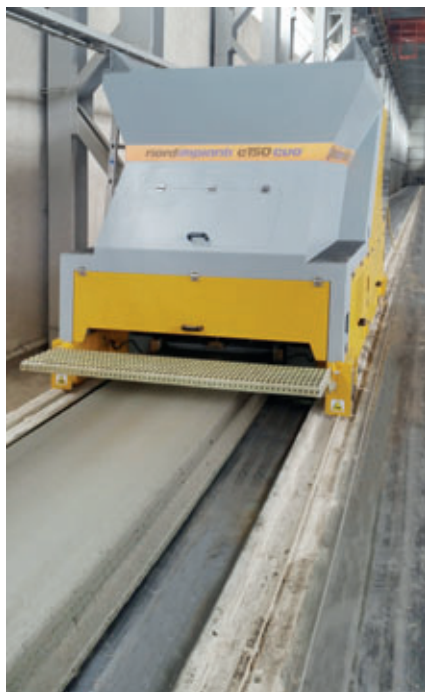
The Extruder machine during the casting phase of a narrow 900 mm wide hollow core slab on a standard 1500 mm wide production bed.
